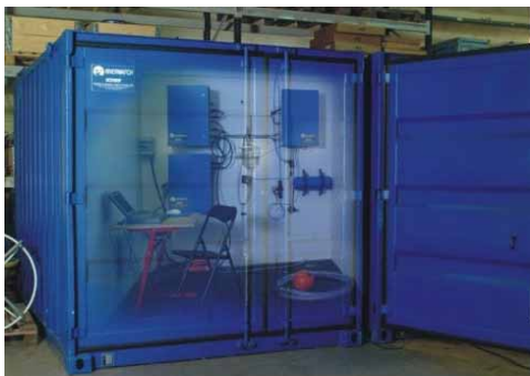
Automatic river station, fixed solution
